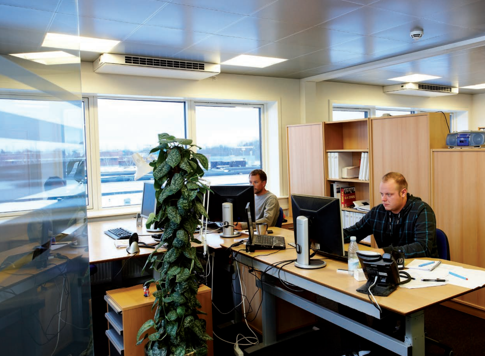
Two AM 300 air handling units are installed in the office, integrated into the ceiling.
